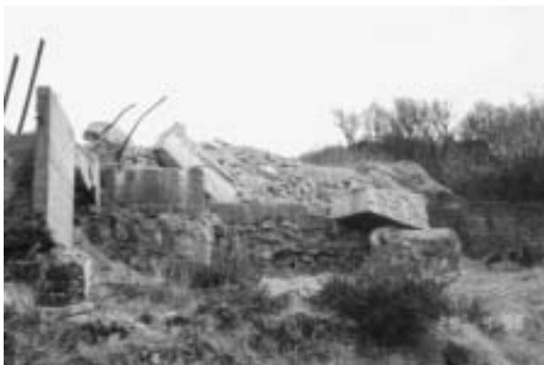
Figure 2: Remains of stone bases with loose blocks and dangerous metal work, Holman's Quarry (c. Kerrier District Council)
