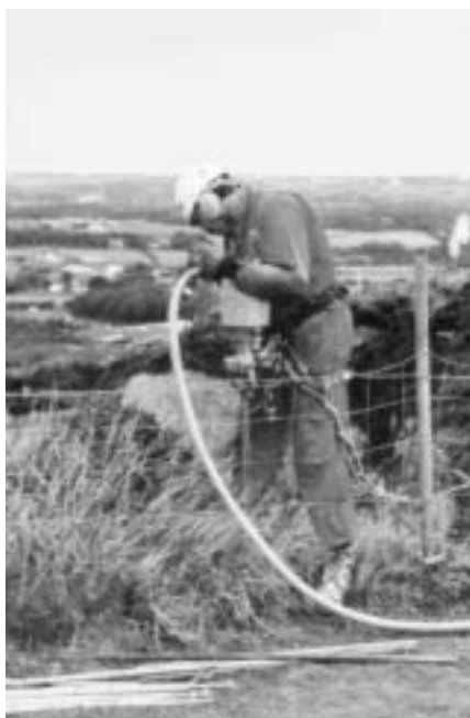
Figure 3: Phase 1: Drilling to erect steel stabilisation mesh at Holman's Quarry (c. Kerrier District Council)
